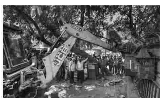
Authorities had issued an eviction notice on Sunday to residents of the locality near the Old Iron Bridge, instructing them to vacate their homes by Monday. The demolition drive, part of the Yamuna beautification project, was scheduled for Tuesday and Wednesday.
